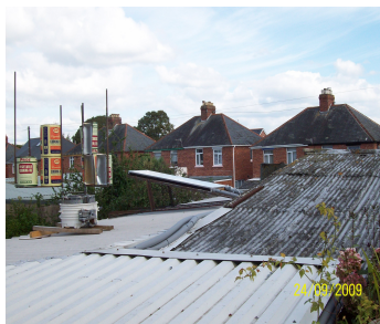
Solar Panel ("wind turbine" previously removed)
